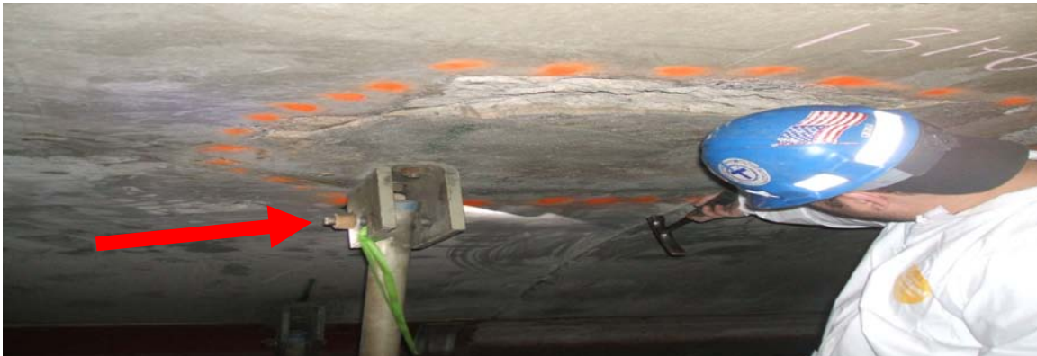
Figure 1. TWT Adhesive Anchor Supporting Ceiling Panels
