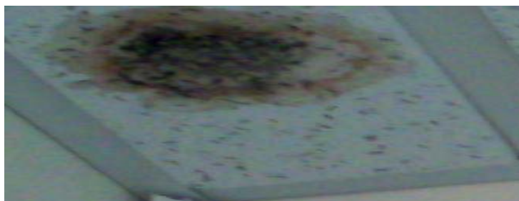
Figure 2. Damage to Ceiling at Washington Center Due to Leaky Pipes
