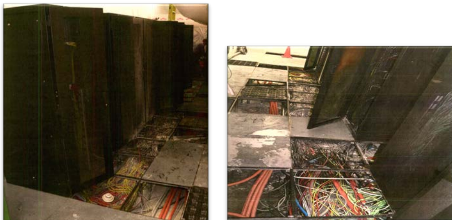
Figure 2. Chicago Center’s Fire Damage
