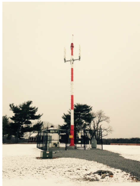
Figure 3. ADS-B Radio Tower and Ground Infrastructure, Frederick, MD
